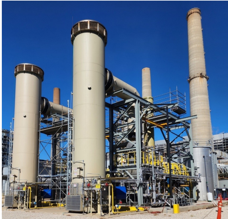
Heartland Concentrator system integrated into plant operations.
